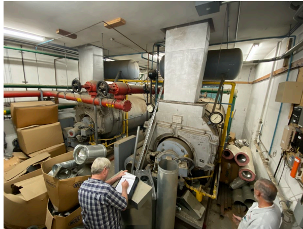
Boiler Room at La Sierra
